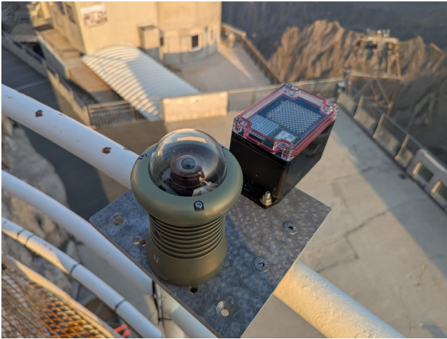
Figure 9 – FRIPON camera and radiometer at Pic du Midi observatory.
